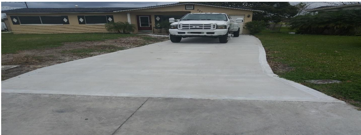
321 Amador Circle Damage Driveway replacement
